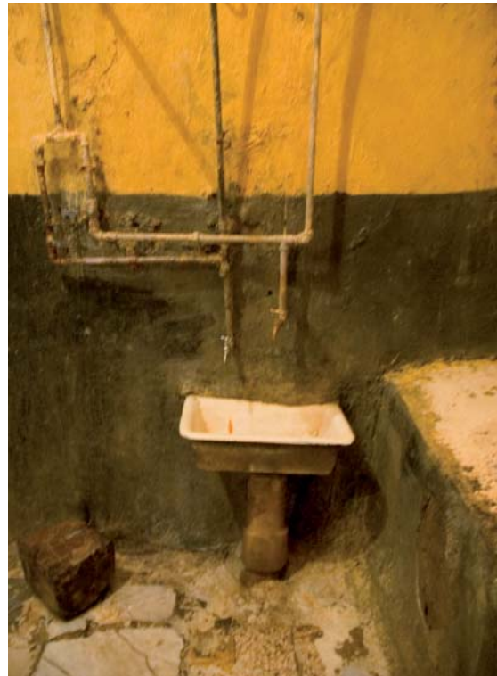
Figure 4 Poor Quality Water Pipes Insensitively Introduced in the Hammām. (Source: Sibley, M- AHRC funded project: Historic Hammāms of North Africa@June 2007).
